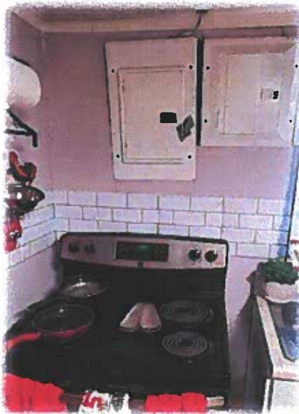
(Safety Hazard Electrical Panels)
