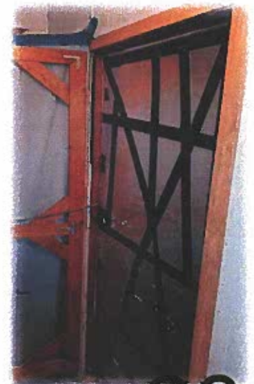
(Safety Hazard Home Entry Door)
