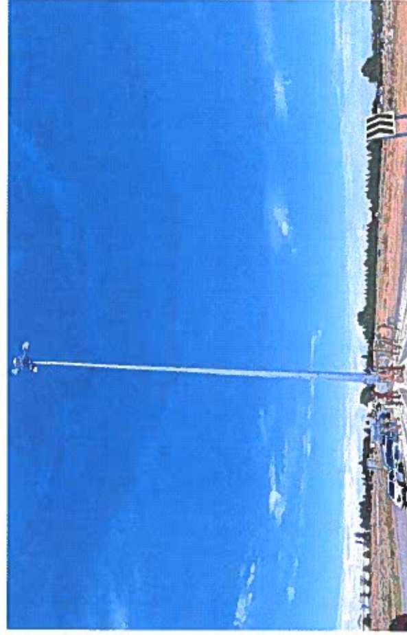
HIGH MAST ILLUMINATION
